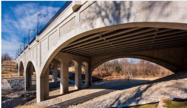
2022 Project Achievement Award | Greater Than $15M Edmondson Avenue Bridge Replacement (Transportation) Baltimore City DOT | JMT
